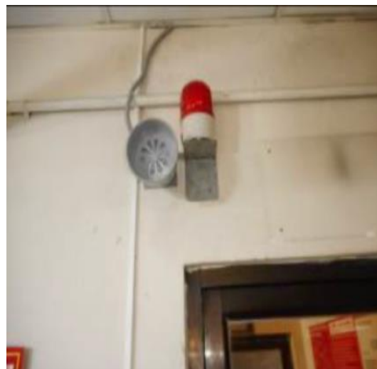
Fire alarm bell
