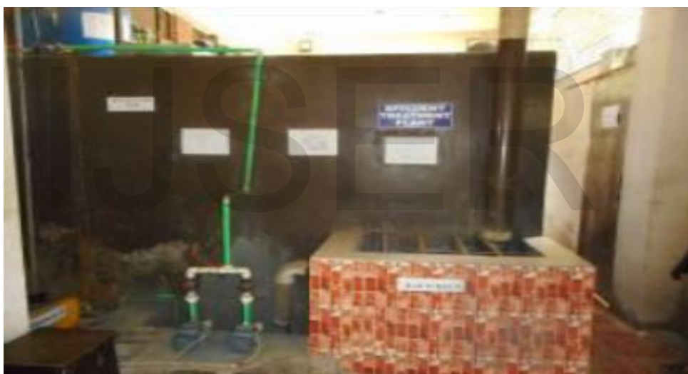
Fig 4.28 Effluent Treatment Plant (ETP)
